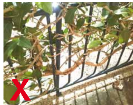
Vegetation that can be used to climb into the pool area should be removed.
